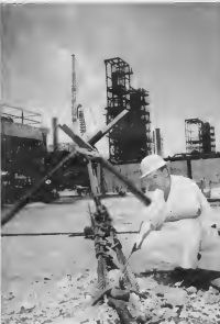
ZONE SUPERVISOR Bill Pea checks guy cables. ZONE SUPERVISOR Bill Pea ta check cableana.
